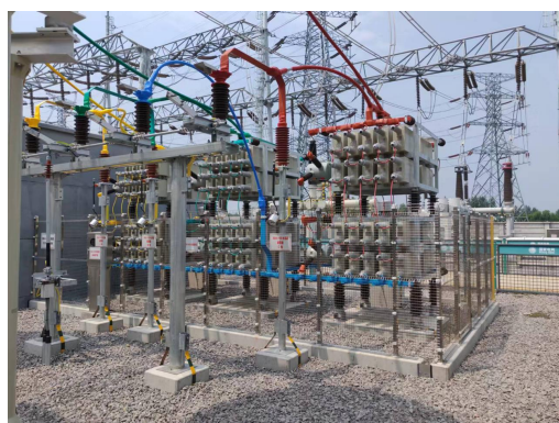
35kV1#B 电容器贮油坑
