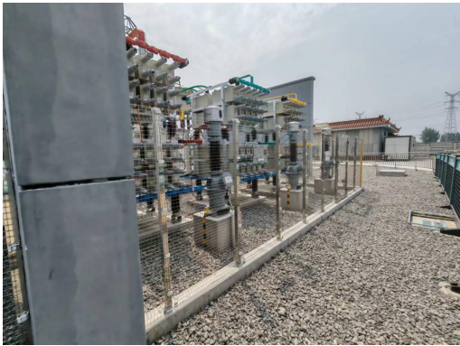
35kV1#A 低压电容器组
