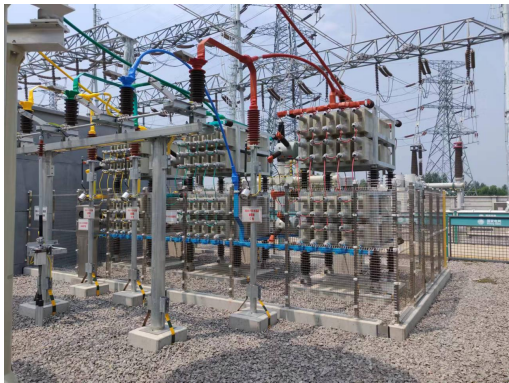
35kV1#B 低压电容器组贮油坑
